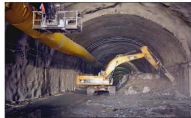
Figure 17. Mechanical excavation of the tunnel bench after blasting. Excavator and hydraulic hammer were used for scaling and rock breaking.
