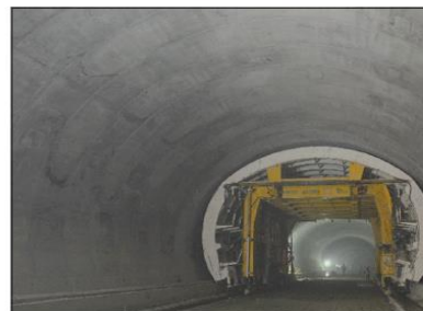
Figure 19. Picture appreciating the Progress of tunnel final lining and the steel form along tunnel alignment
