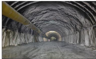
Figure 16. Tunnel excavation with rock condition from fair to good. Steel fiber shotcrete and rock bolts are shown as primary support.
