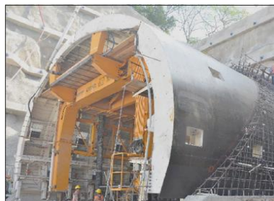
Figure 18. Tunnel lining operations by Brisamar Portal. Steel form is ready for the first concrete pouring as steel rebar reinforcement is installed.
