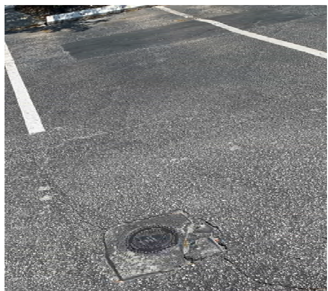
Site – 68 Ciccio Water Restaurant Monitoring well in site parking lot (facing east)
